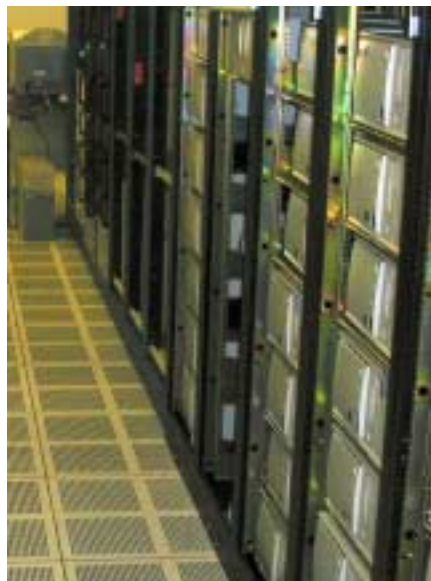
Figure 5. Data Center Racks
